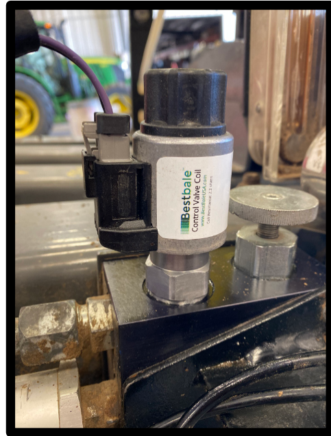
Install BestBale valve & coil Plugs into X12
